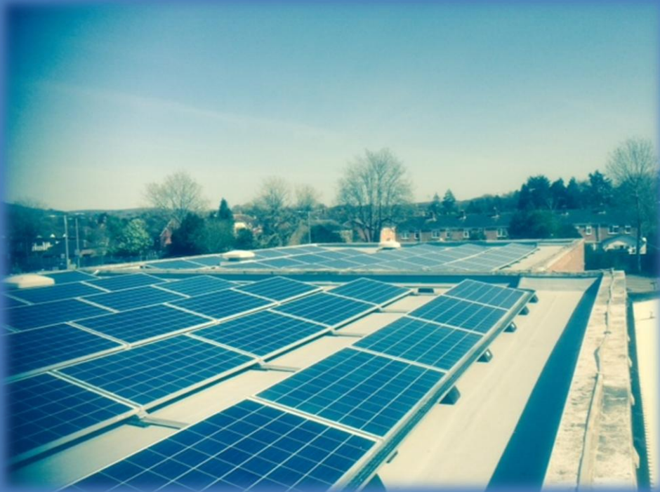
Cranleigh Leisure Centre 18kW solar PV array
